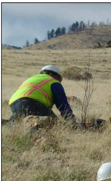
Hand planting of native shrubs at the Arrowcreek Restoration site in Washoe Valley
