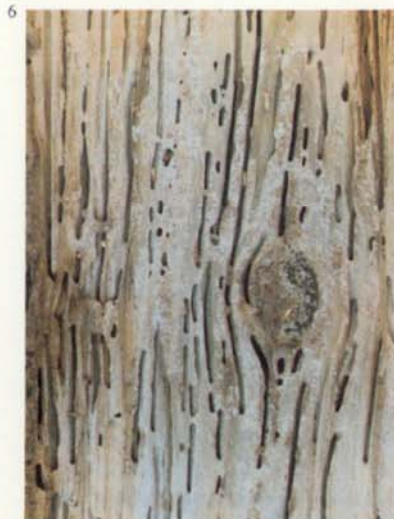
Figure 6. — Surface of wood removed to show damage done by termites and the specks of excrement on the gallery walls.
