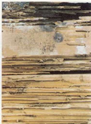
Figure 7. — Wood attacked by subterranean termites has a honeycombed appearance because the workers tunnel along the softer grain of the wood.
