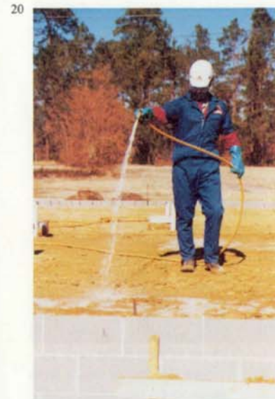
Figure 20. — Chemical treatment of the fill material prior to pouring a concrete slab protects wood in the building from termite attack.
